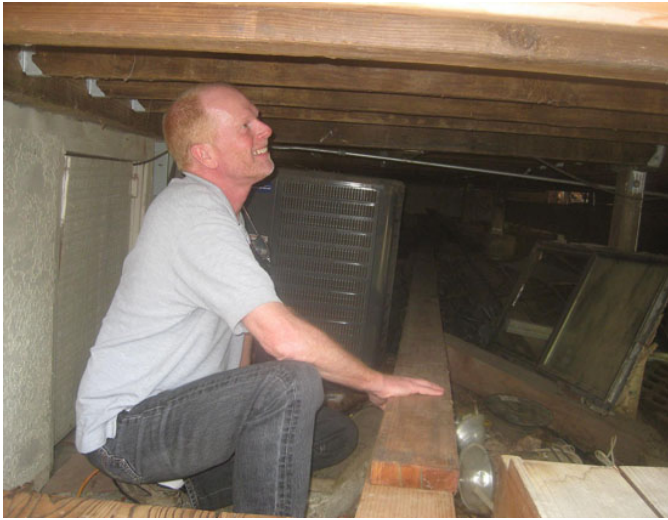
Houghton inspects the under-story of a deck for dry rot. Photos Chris Lavin
