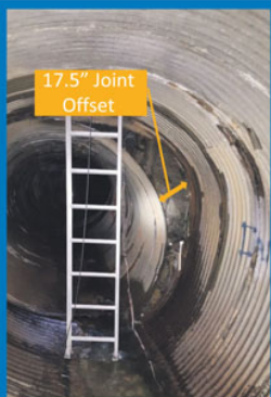
Figure 9: Joint Offset of CMP at Sinkhole Location
