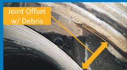
Figure 8: Joint Offset with Debris Intrusion 4/27/16
