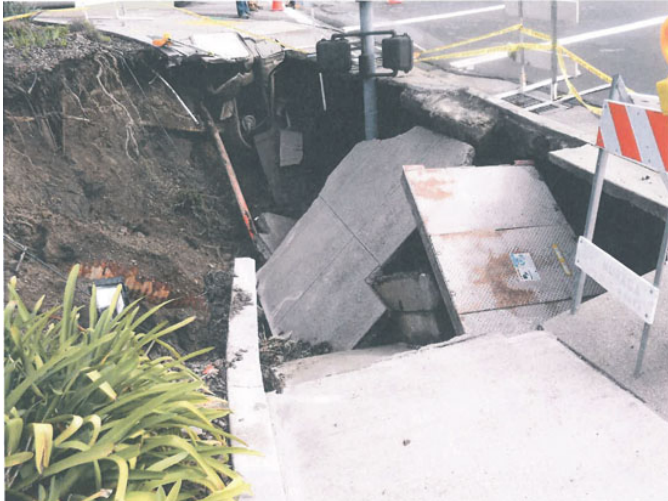
Monday, March 14: A traffic signal pole, a PG&E electrical switch vault and portions of the sidewalk collapsed into the sinkhole. Photos provided
