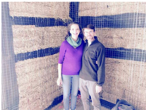
Amber and Norman Remer smile inside their house of straw, while under construction. Photo John T. Miller
