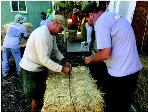
From left: Architect David Arkin and contractor Keith Kuhlmann at the straw house building site. Photos provided
