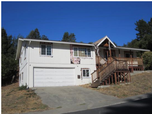
A state of disrepair at 90 Greenfield Dr. Photo Vera Kochan
