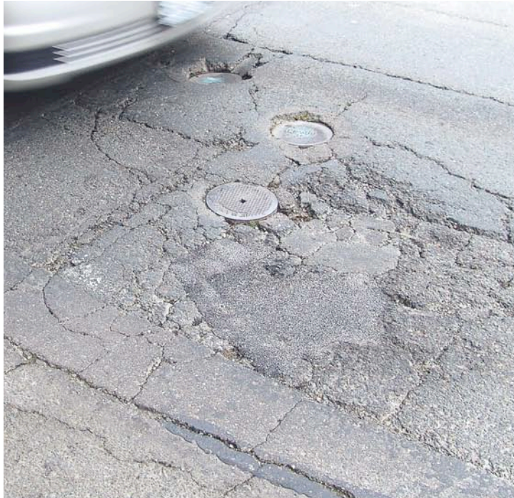
Rough road conditions on Moraga Way
