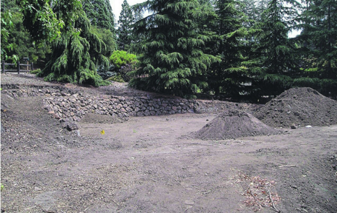
Ground has been broken for an outdoor labyrinth at St. Stephen's Episcopal Church, Orinda.
