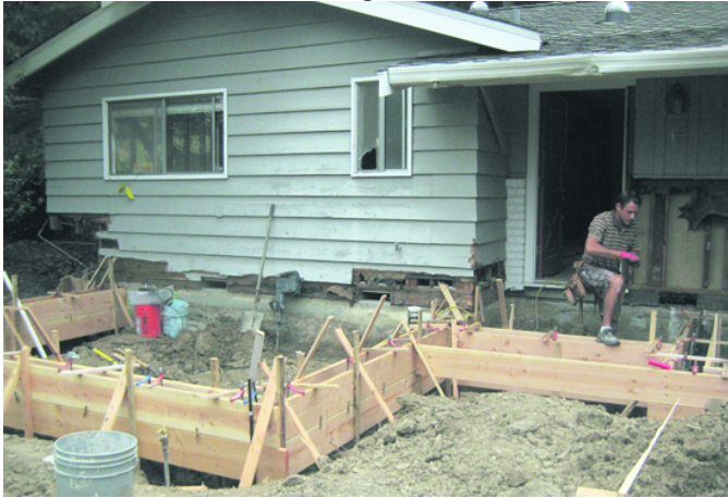
Daniel Leleu builds a new foundation at the front of the home.
