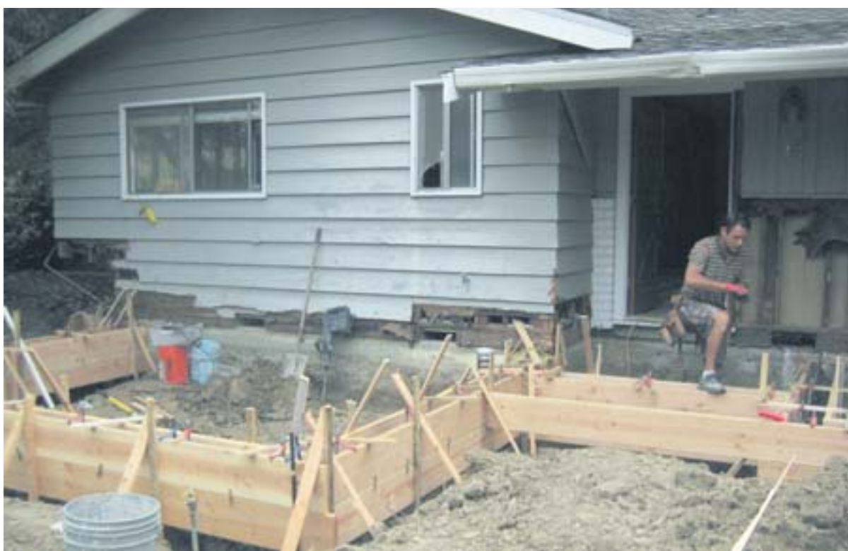
Daniel Leleu builds a new foundation at the front of the home.
