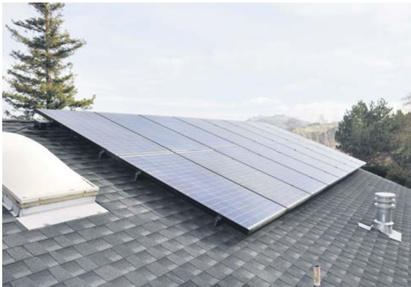
The biggest of our three solar panel arrays holds 16 of the 32 panels.
