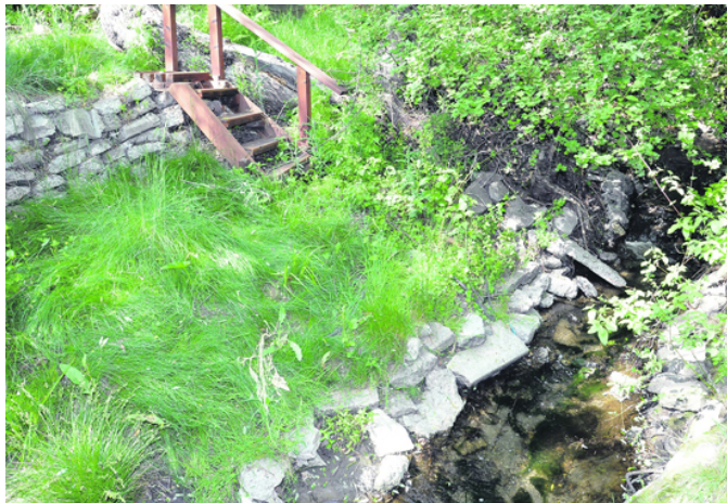
A simple flight of stairs built by Tom Preston accesses the creek bank planted with native grasses.
