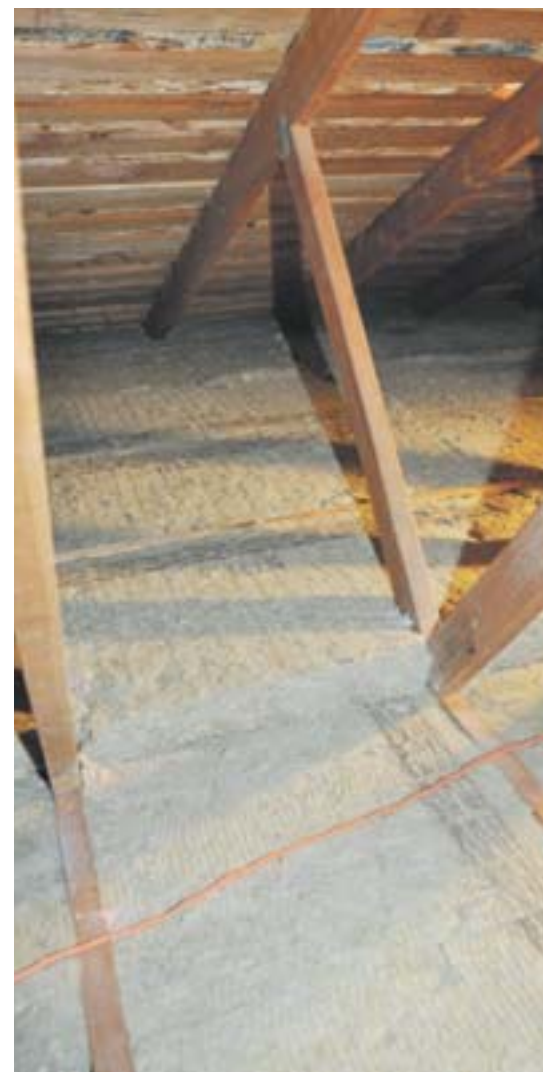
Two perpendicular layers of stone wool insulation batts were easy to install in this Moraga home.
