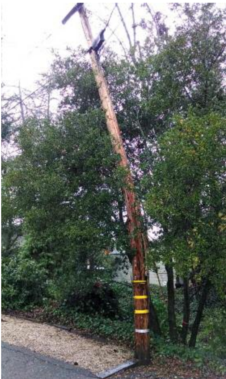
A damaged power pole after recent storms
