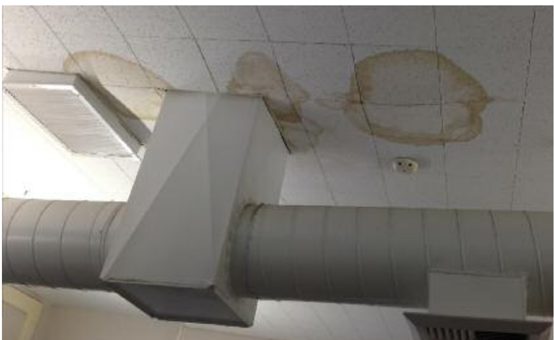
Ceiling water damage at a Lafayette school.
