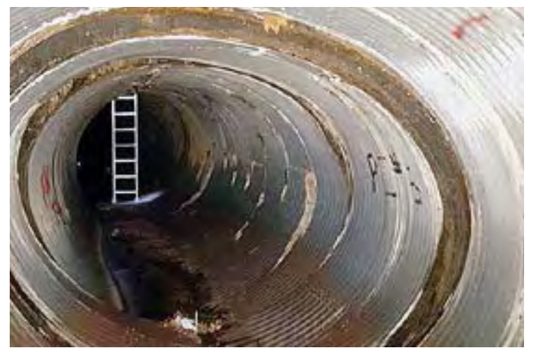
Pipe Crown Deformation
