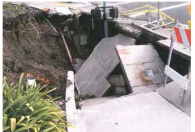
Monday, March 14: A traffic signal pole, a PG&E electrical switch vault and portions of the sidewalk collapsed into the sinkhole. Photos provided
