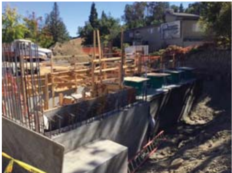
The new Diablo Vista pumping plant. There is great news for traffic on Mount Diablo Boulevard in Lafayette: East Bay Municipal Utility District's contractor has almost finished installing a 30-inch diameter pipeline and related service lines at the southwest corner at Mt. Diablo Court, next to the cemetery.
