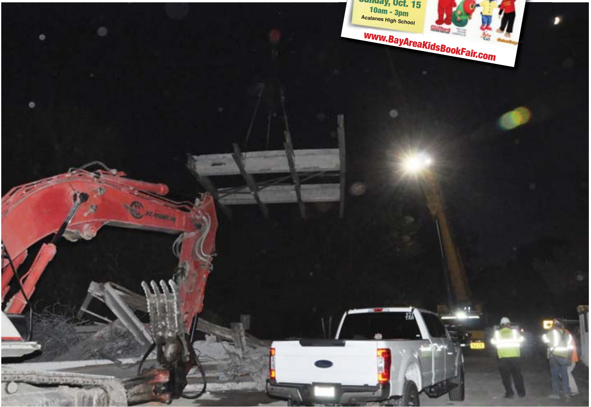
The dismantling of the Canyon Bridge continued after darkness fell on Sept. 26. Photo Andy Schreck
