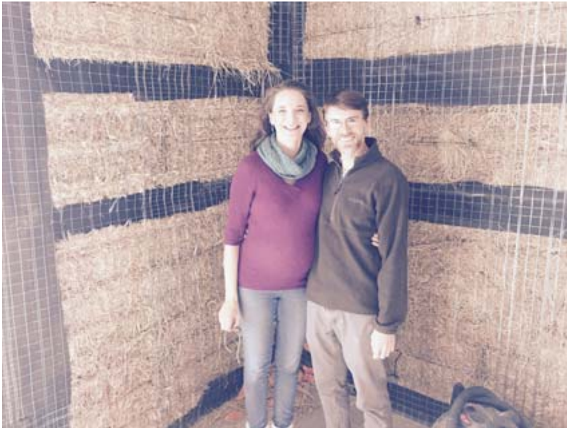
Amber and Norman Remer smile inside their house of straw, while under construction.
