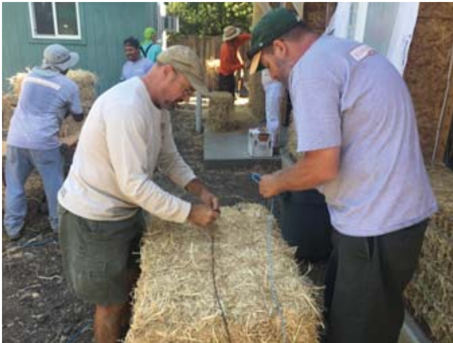
From left: Architect David Arkin and contractor Keith Kuhlmann at the straw house building site.
