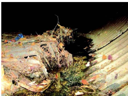
A broken pipe eight feet upstream at Rheem Boulevard and Center Street Photo provided
