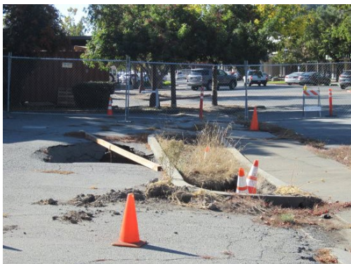
Rheem sinkhole gets larger Photo Vera Kochan
