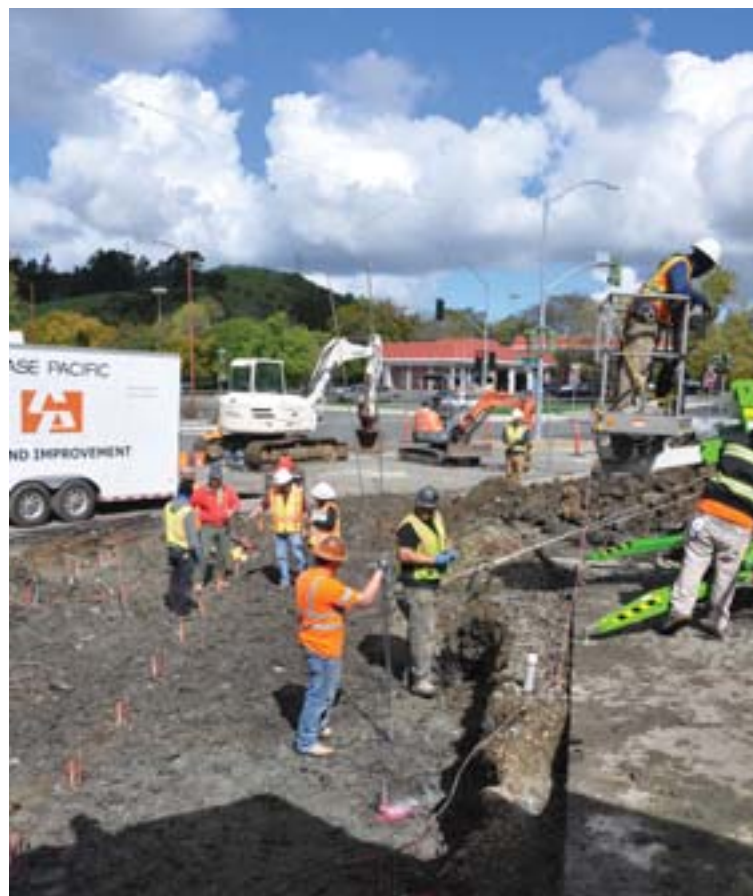
Work on the Moraga sinkhole at the corner of Rheem Boulevard and Center Street is in progress. Cars are allowed to enter but not exit the shopping center from Rheem Boulevard.
