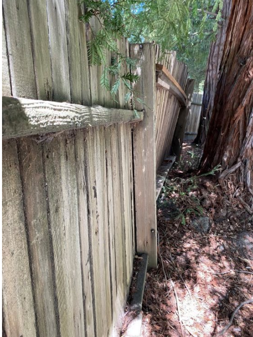
Hacienda fence beyond repair Photo courtesy Parks and Rec
