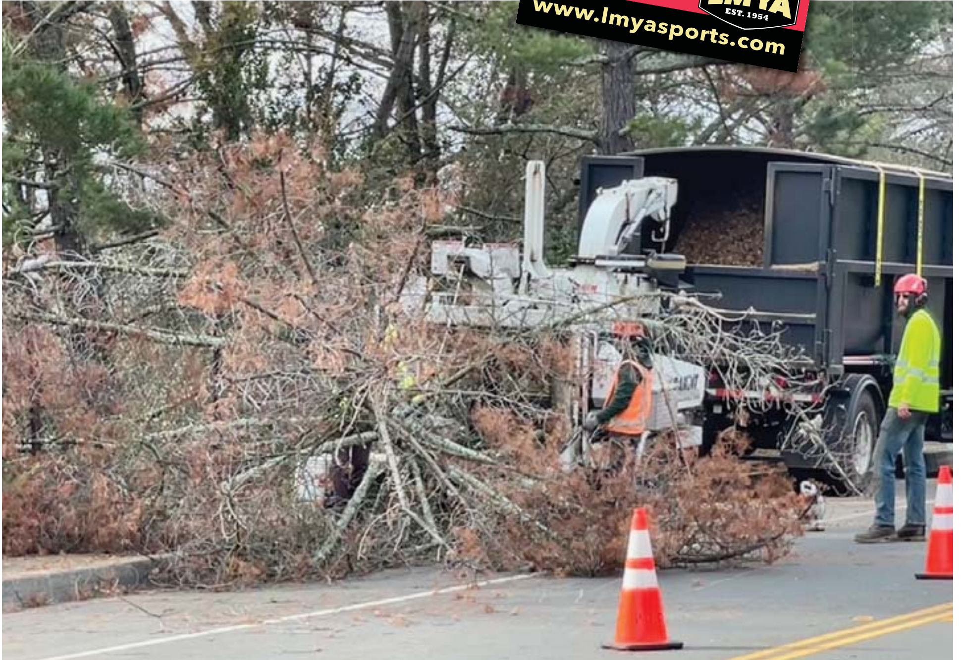
Recent tree mitigation work being done by Caltrans on Highway 24 near St. Stephens Drive, on El Miso Ranch Road.
