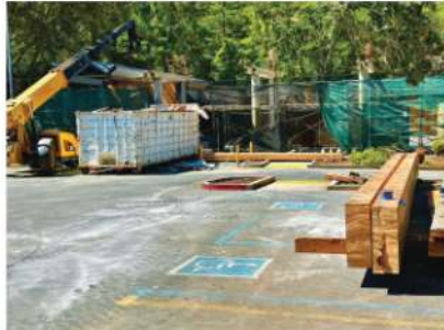
Construction has begun on the transformation of the old Bank of America building in downtown Orinda.
