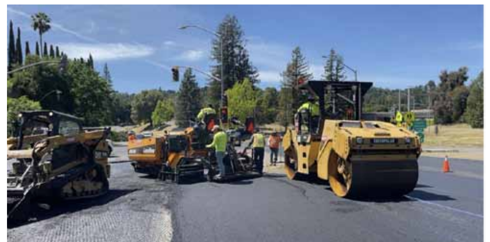
Mt. Diablo Boulevard paving at Acalanes Road and SR 24 on- and off-ramps
