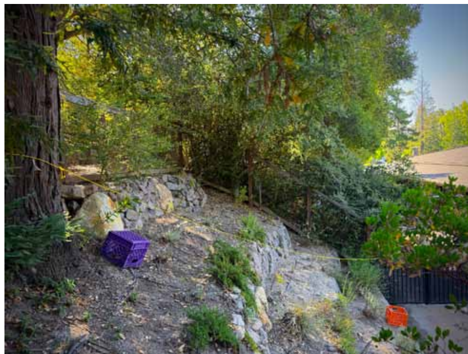
The yellow rope indicates roughly where the retaining wall will be built for Vista Verde Senior Housing. This corner has been used as part of the outdoor classroom by The Orinda Preschool.
